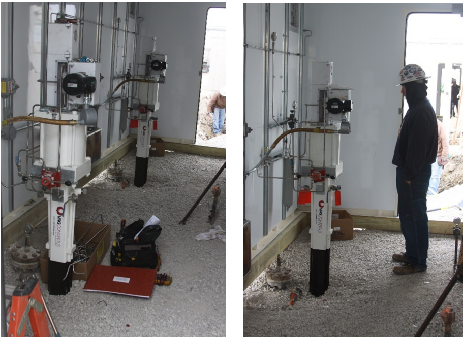
Figure 1 – Below Ground Control Valve Installation
